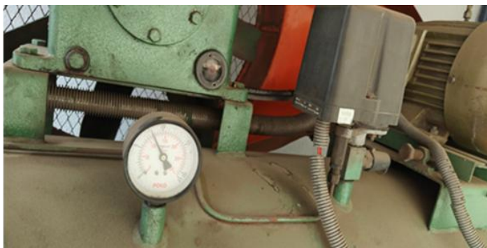
Compressors for Purging in the Tank
